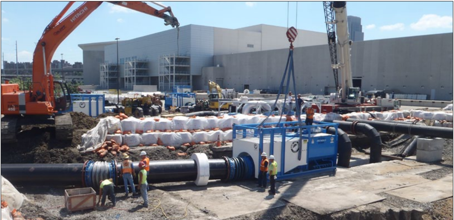
Rain for Rent crews install the first FP-1050 42" Axial Flow floating pump into the newly constructed temporary CSO suction pit.
