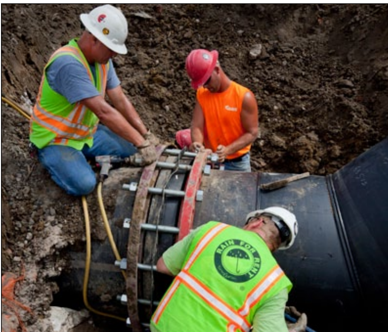
A section of 42 inch HDPE discharge line for pump station 2 is bolted into place. This line was fed by a FP-1050 capable of 68,500 gpm.
